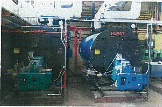
Figure 4-42: Water Treatment Plant Boilers
