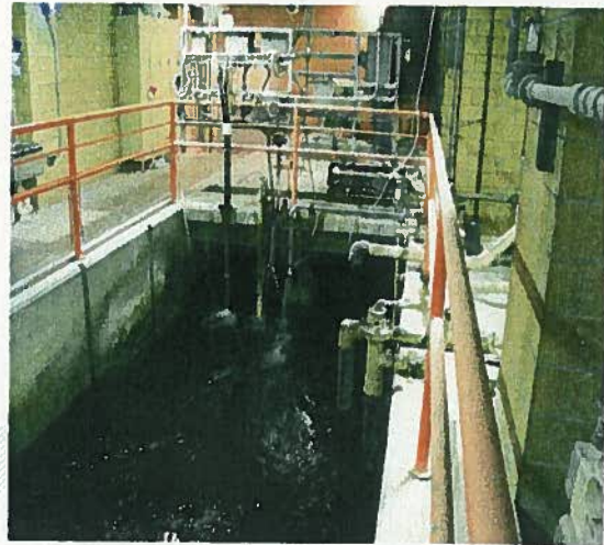
Figure 4-13: Rapid Mix Channel
