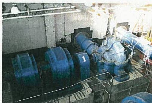
Figure 4-25: High Service Pump
