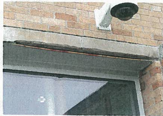
Figure 4-38: Deterioration around Windows
