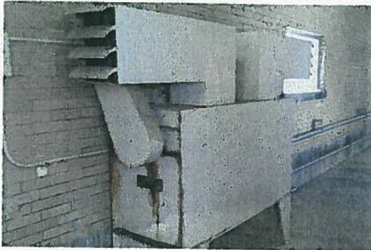
Figure 4-43: Water Treatment Plant HVAC
