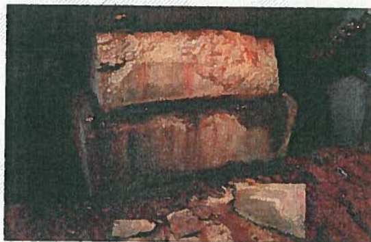
Figure 4-34: High Service Pump Station Pipe Supports
