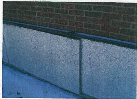
Figure 4-36: Aggregate Covered Panels
