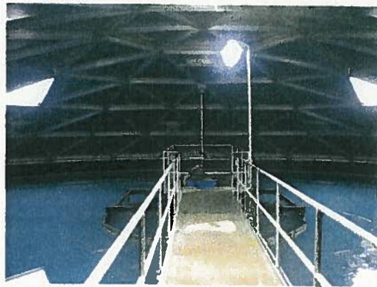
Figure 4-27: Dewatering Facility Thickener
