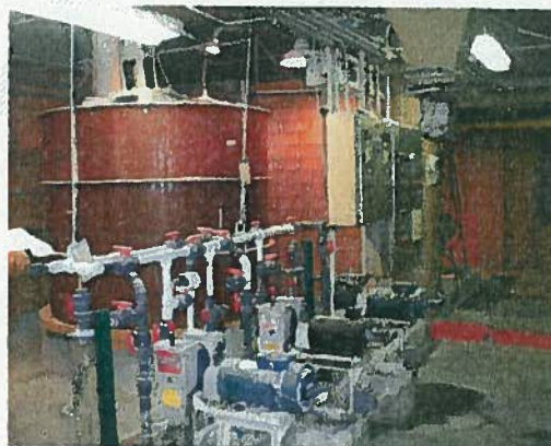
Figure 4-21: Polyphosphate Storage and Feed System
