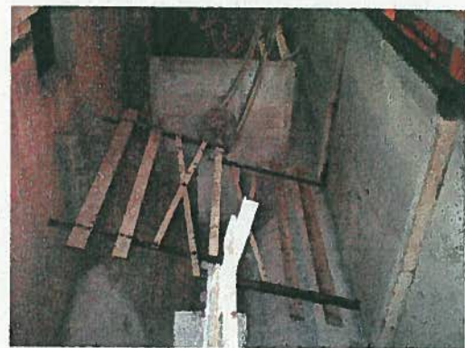
Figure 4-14: Horizontal Flocculator Paddles
