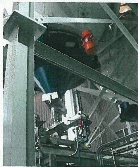
Figure 4-17: Permanganate Feed System
