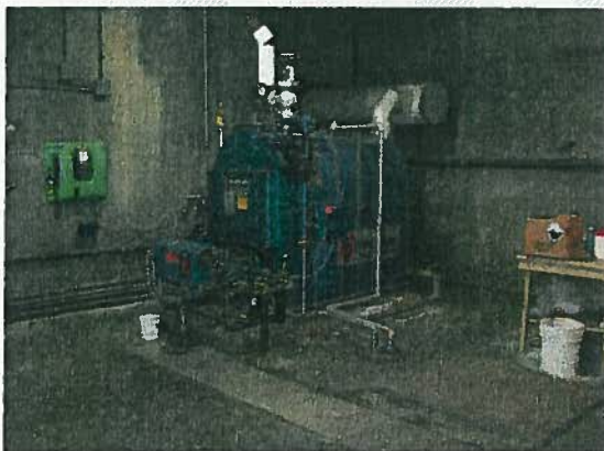
Figure 4-40: Low Service Pumping Station Boiler
