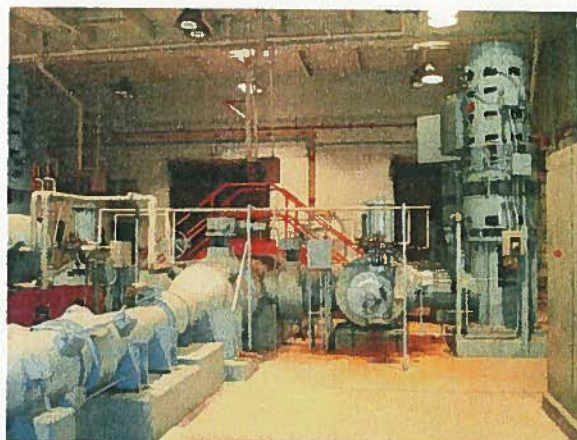
Figure 4-31: Heatherdowns Pump Station
