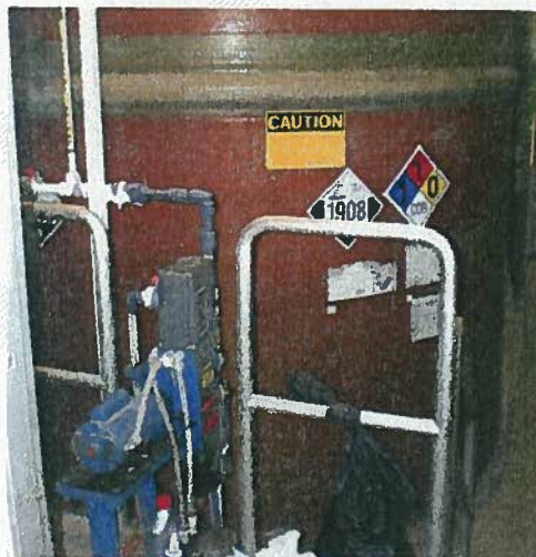
Figure 4-24: Chlorine Dioxide Generation System
