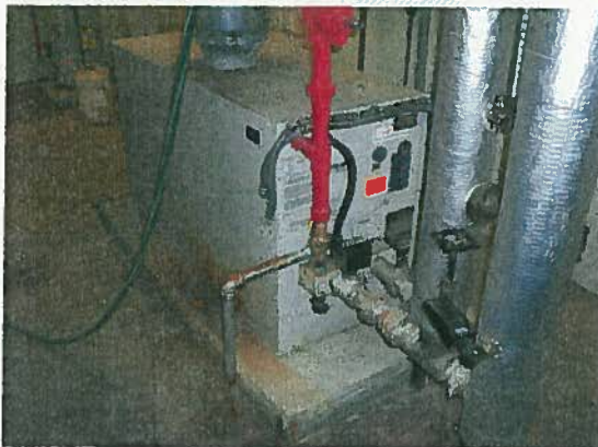
Figure 4-44: Residuals Handling and Dewatering Facility Boiler
