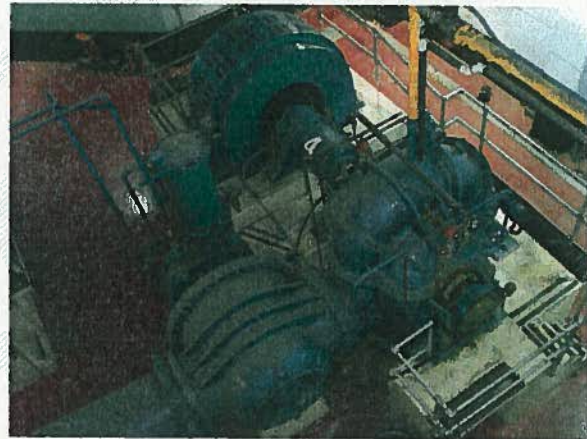
Figure 4-10: Low Service Pump
