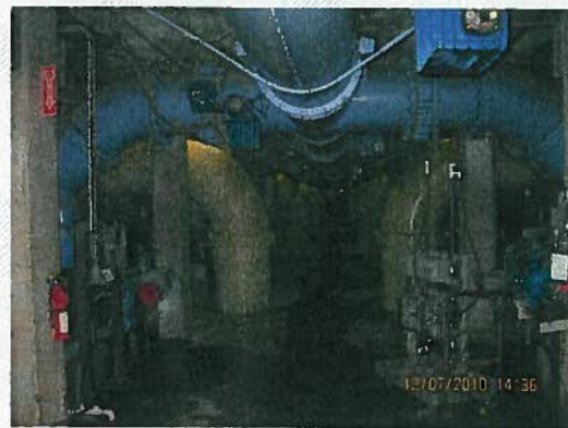
Figure 4-16: Filter Pipe Gallery
