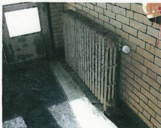
Figure 4-41: Radiator in Low Service Pump Station
