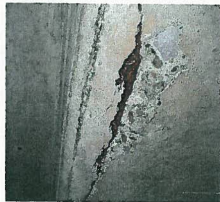
Figure 4-39: Deterioration in Tunnels
